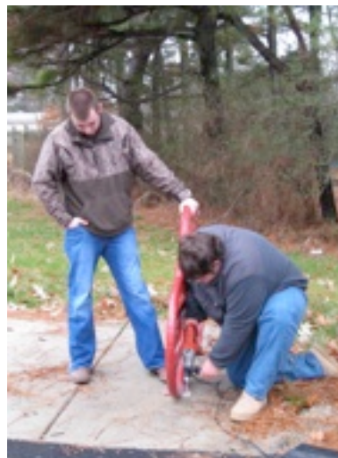
Students from the NEA Career and Technical Center install the first of several new bicycle racks along the Jonesboro Greenway
